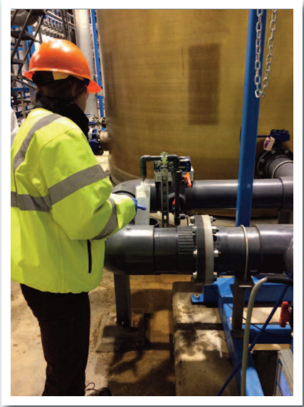
CEMP Field Technician Abby Debiak sampling effluent at the Humboldt Mill Wastewater Treatment Plant.
