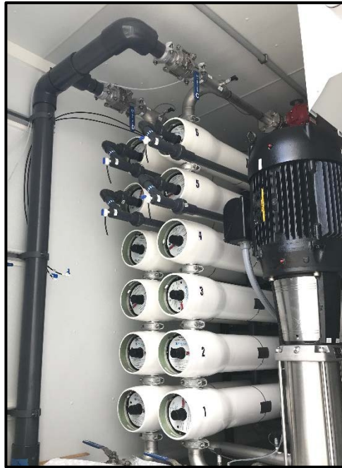
Water Treatment Plant, Reverse Osmosis Unit
