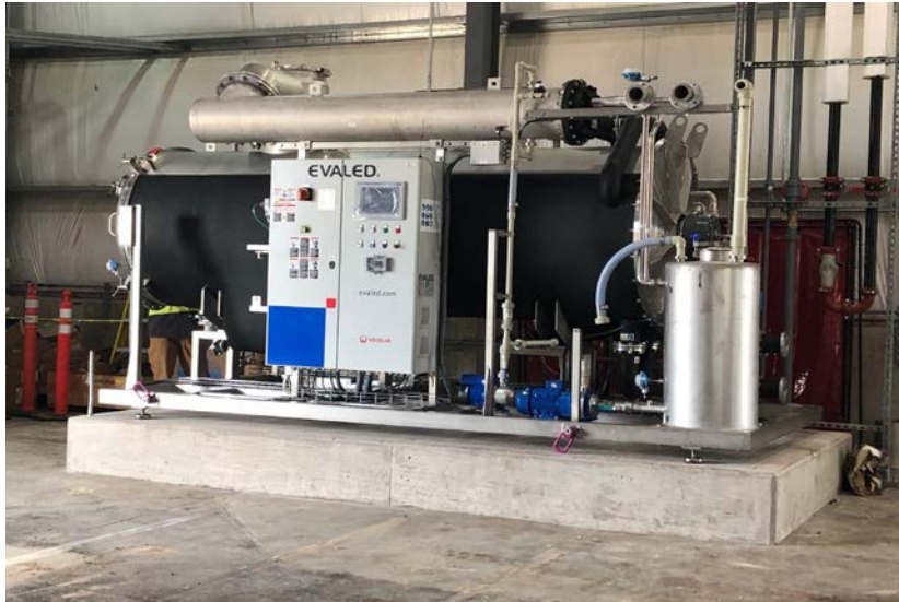
Crystallizer installation, August 2020
